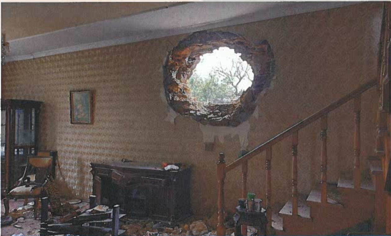
Valeriy's home was hit by a rocket on 3 April, 2022.
