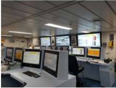
Main Control Room
