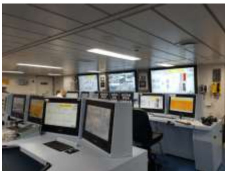
Main Control Room
