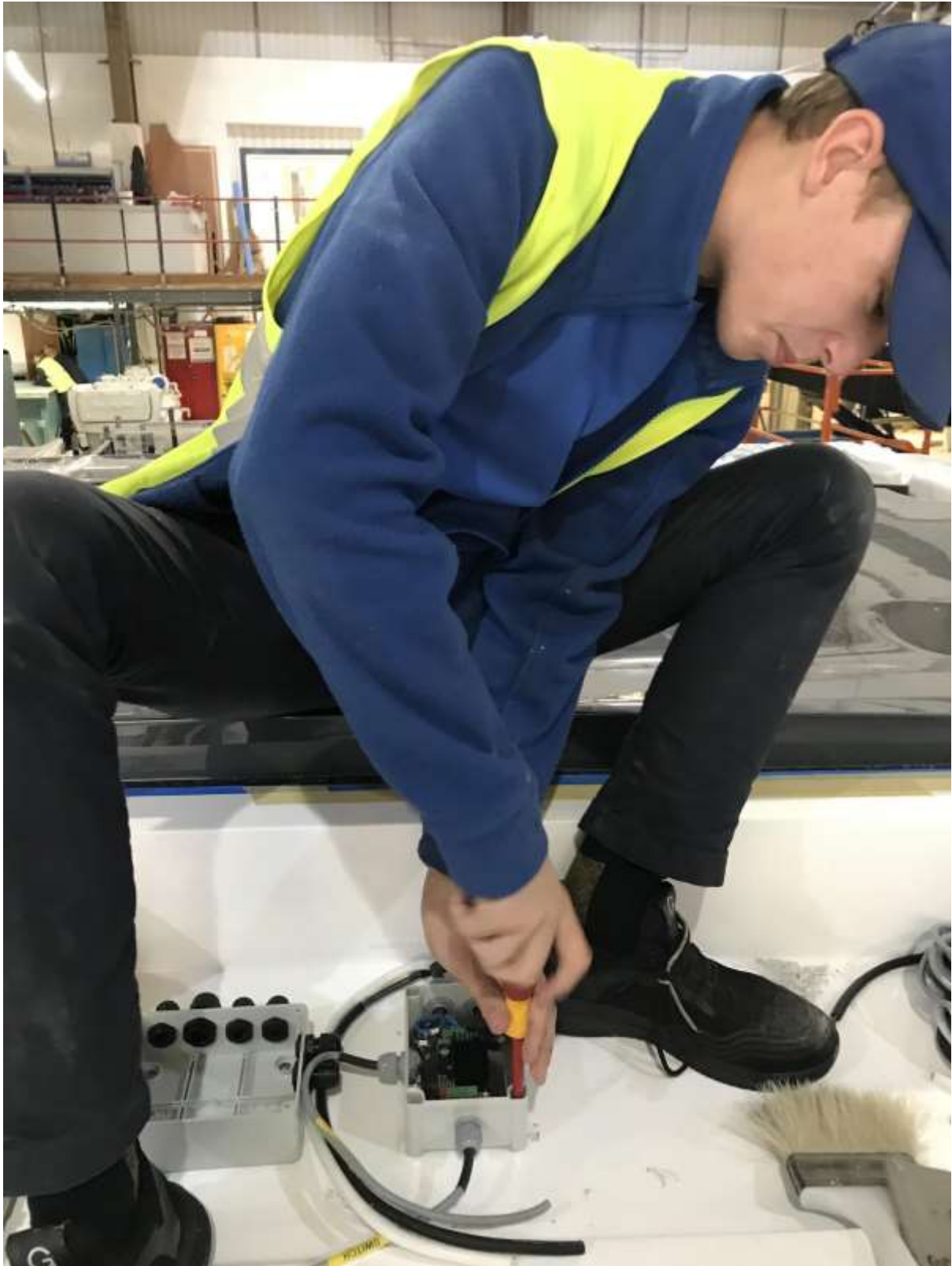
These images are showing some of the work I have been doing where I am completing the wiring of a control box and motor of one of the roof systems we work on.
